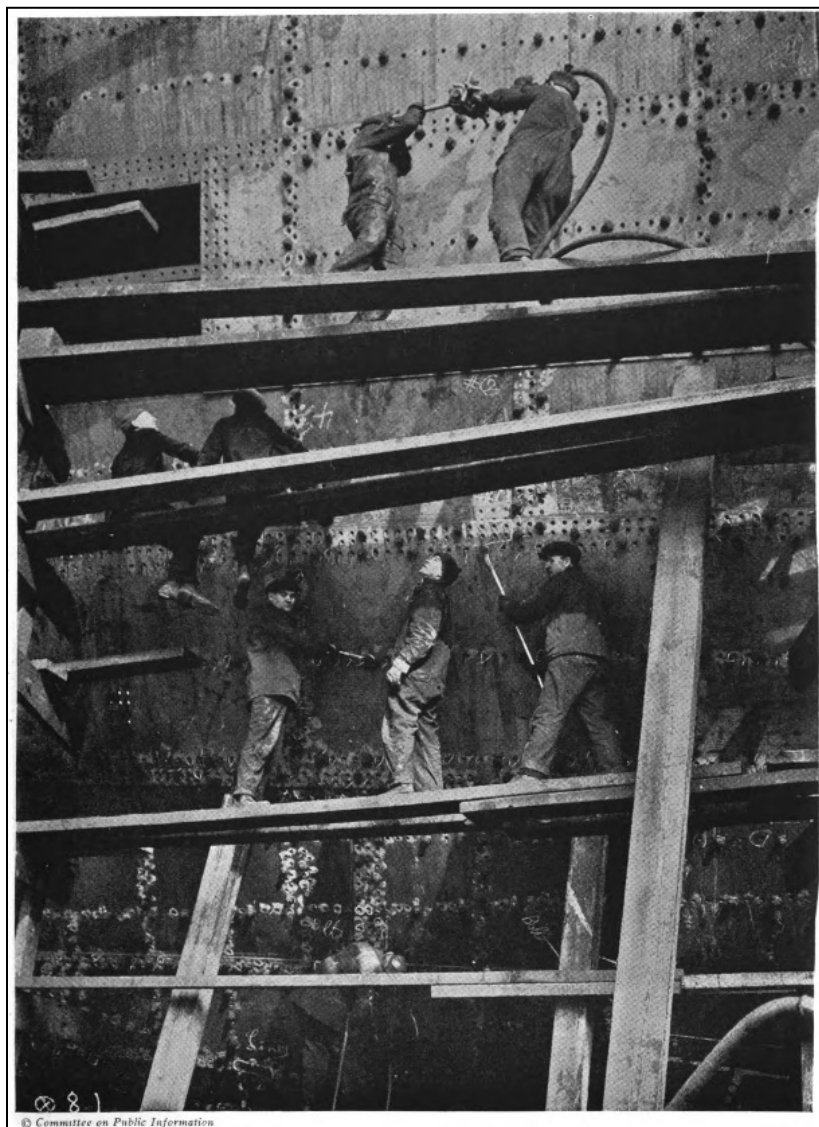
Figure 7-71 Workers at the American International Shipbuilding Corporation's Hog Island Yard assemble standardized, pre-fabricated merchant vessels.
