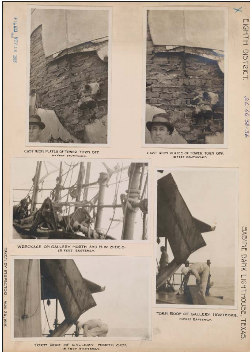
Figure 84. Sabine lighthouse damage in eight service photographs taken 24 August 1915. (Courtesy of NARA.)
