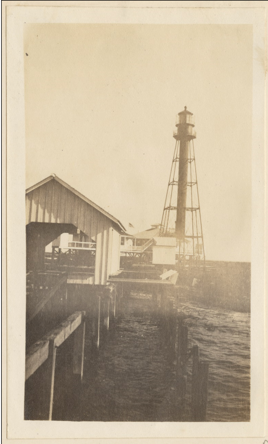
Figure 86. View of Chandeaur Light Station wharf damaged during July 1916 hurricane. (Courtesy of NARA.)
