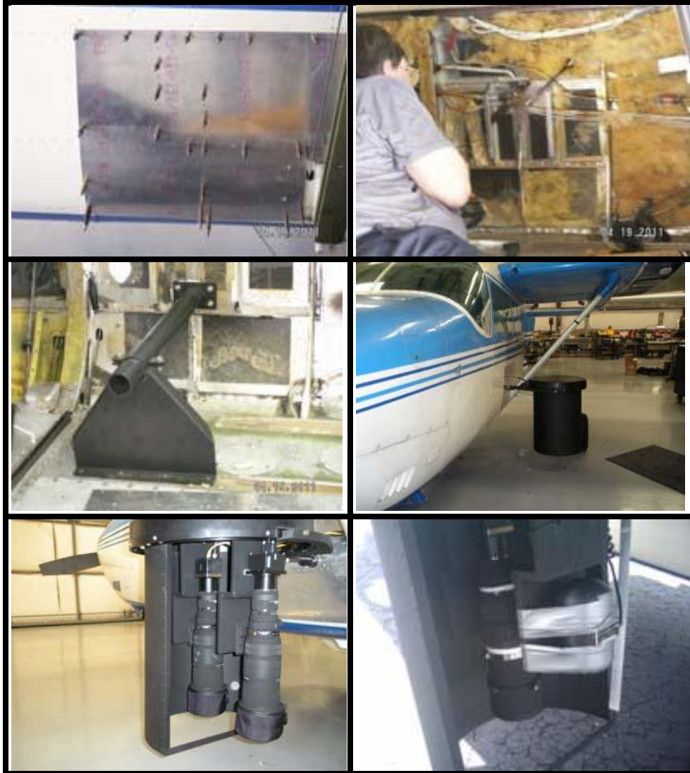
Figure 2–3. Installation of camera mount system on the Cessna 337 Skymaster in Raleigh NC prior to Operations House, showing external airframe reinforcement plates and camera mount attachment bolts (top left), camera interior in preparation for mount installation (top right), inner mount axle and support strut (middle left), and fully installed mount with windshield (middle right), rear view of fully installed mount system with two mounted cameras (bottom left), and gyrosopic stabilizer installed during final week of Operations House experimental flights (bottom right).
