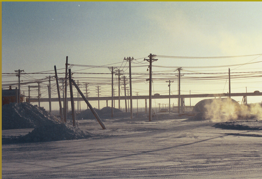
Power lines built by the U.S. Navy are used by Barrow Utilities and Electric Cooperative
